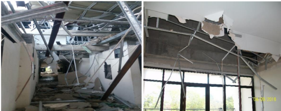
Fig. 4 – Example of architectural damage caused by the earthquake: Ceiling damage due to the falling of the material above it at the rental low-cost housing flats
