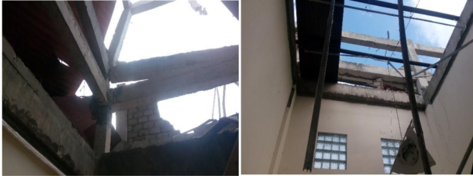
Fig. 3 – Example of major damage to structure caused by the earthquake: Crushing at beam-column joints at the North Lombok Police Station housing flat
