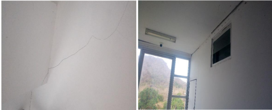
Fig. 5 – Example of minor damage caused by the earthquake: Hairline Cracks on the wall and falling of ceiling list at Sumbawa Technology University flats
