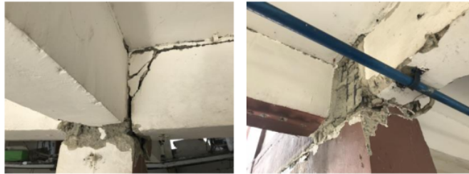
Fig. 8 – Damage of beam-column joint due to earthquake
