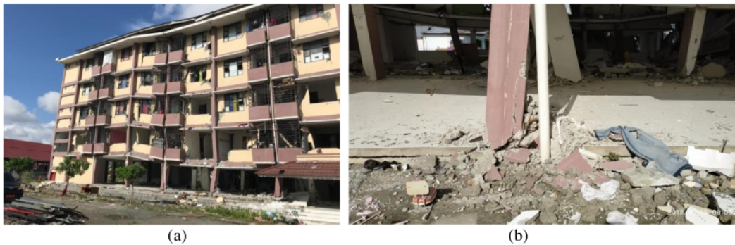
Fig. 5 – Structural damage: (a) compression failure in column, (b) tensile-shear failure in column
