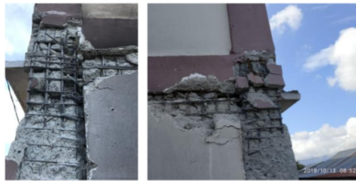
Fig. 9 – Stirrups installed properly in column, beam and joint, concrete crushing because of tension
