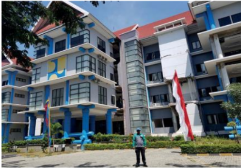
Fig. 2 – Damage in the Front of the Building
