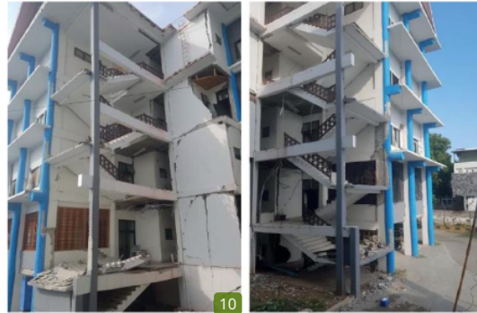
Fig. 3 – Damage in the Back of the Building
