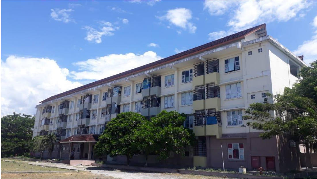
Fig. 2 – Front view of damage occurred on rental low-cost housing flat UPT Dinas PU Palu
