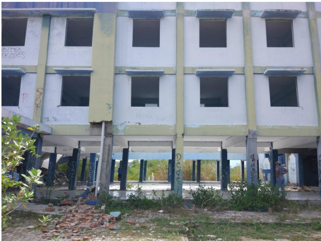
Fig. 3 – Front view of damage occurred on rental low-cost housing flat Univ. Tadulako
