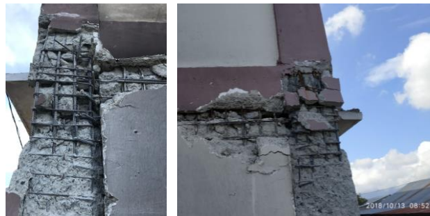
Fig. 9 – Stirrups installed properly in column, beam and joint, concrete crushing because of tension
