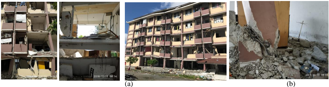
Fig. 1 – Pictures of damaged rental low-cost housing flat Lere: (a) major architectural damage, (b) major structural damage concentrated on base columns undergone compression failure and combined shear and tensile failure
