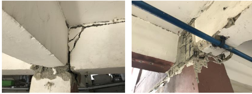
Fig. 8 – Damage of beam-column joint due to earthquake
