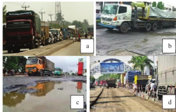
Fig. 2. Condition of Pantura Lane Roads with (a) Heavy Traffic (b) Excess Load (c) Road Damages (d) Routine Maintenance Yearly
