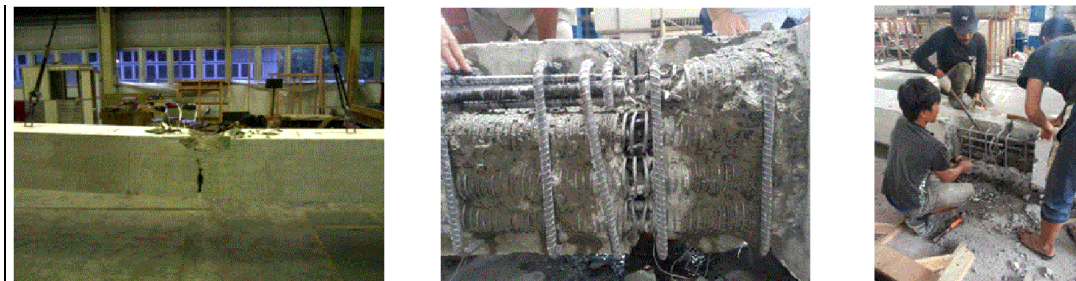
Fig. 14 – Repair of precast segmental hybrid beam and connected with new dissipater ( A_s/A_s'=1.14 )
