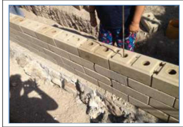
Figure 3 Arrange the walls of the building and prepare the iron for the column
