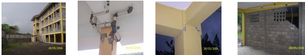
Figure 3.3. Typical damage of soft story effect caused by Yogyakarta earthquake
