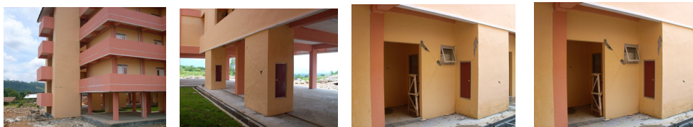
Figure 3.4. Typical damage of soft story effect caused by West Sumatra earthquake
