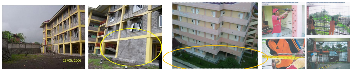
Figure 8.1. Steel bracing and concrete wall strengthening of low cost housing at moderate to high risk zone
