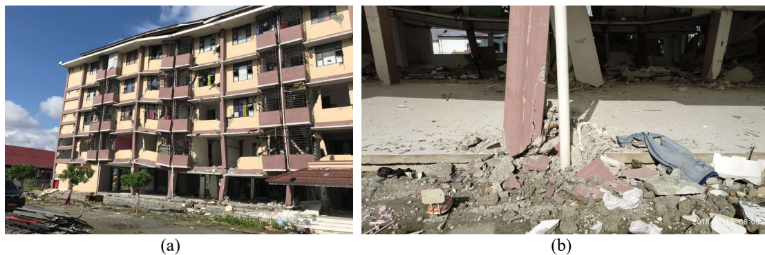
FIGURE 5. Structural damage: (a) compression failure in column, (b) tensile-shear failure in column
