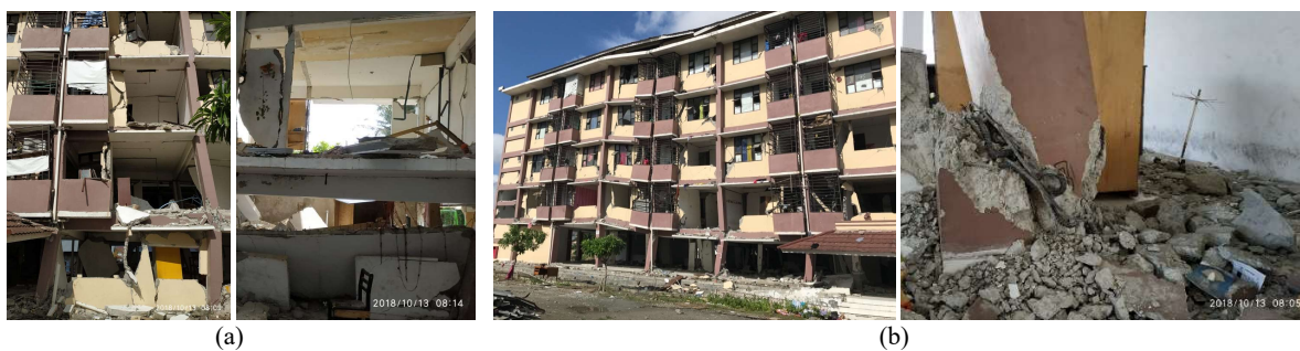
FIGURE 1. Pictures of damaged rental low-cost housing flat Lere: (a) major architectural damage, (b) major structural damage concentrated on base columns undergone compression failure and combined shear and tensile failure
