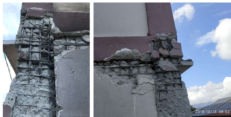
FIGURE 9. Stirrups installed properly in column, beam and joint, concrete crushing because of tension
