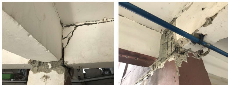
FIGURE 8. Damage of beam-column joint due to earthquake
