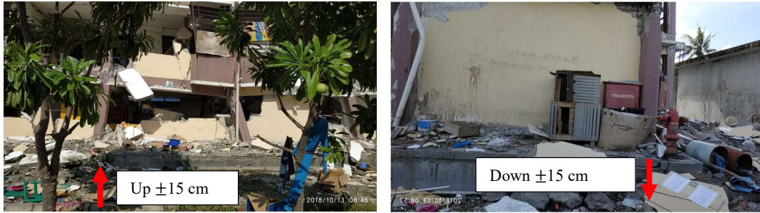
FIGURE 2. Soil deformation pattern due to vertical earthquake (pictures continuous along the length of building)
