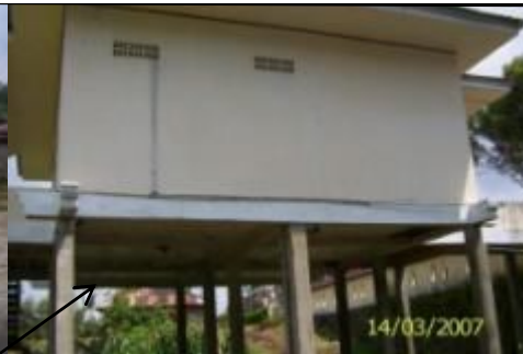
Kegagalan akibat soft storey effect
