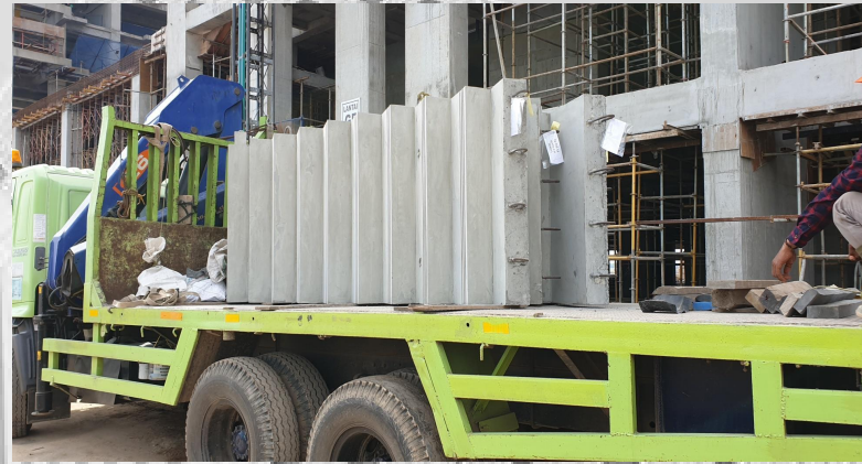
Precast Stair Case
