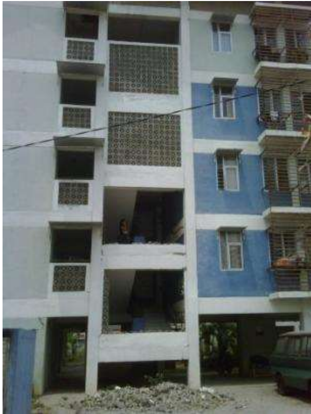
This building have soft story effect (old design before 2008)
