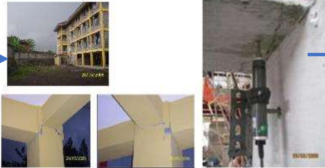
This building have soft story effect (old design before 2008) Yogyakarta 27 Mei 2006
