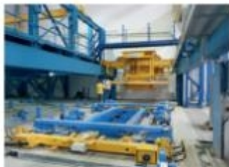
Commissioning of the concrete distributor in KIn - a completely new precast plant is being erected here for the production of sandwich walls as well as solid wall and floor elements.
