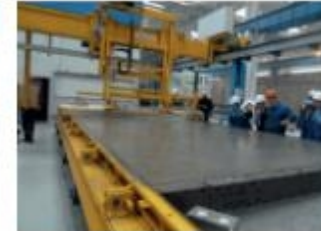
The leveling beam is used to tow up the freshly discharged concrete.
