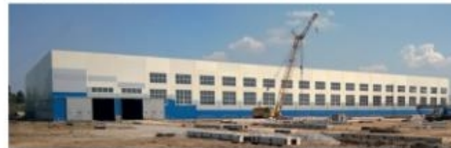
In the new workshop of OOO "EMERCONOMISHY" in Novosibirsk, a production plant is being built consisting of two production plants, reinforcement production with a mesh welding machine, a new bucket truck and a mixing/recycling plant.
