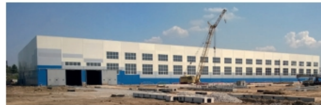
In the new workshop at OOO "ENERGOMONASH" in Novosibirsk, a production plant is being built consisting of two circulation plants, reinforcement production with a mesh welding machine, a new bucket robot and a mixing/recycling plant.
