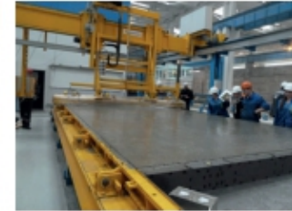
The leveling beam is used to travel up the freshly discharged concrete.
