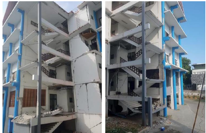
Fig. 3 – Damage in the Back of the Building
