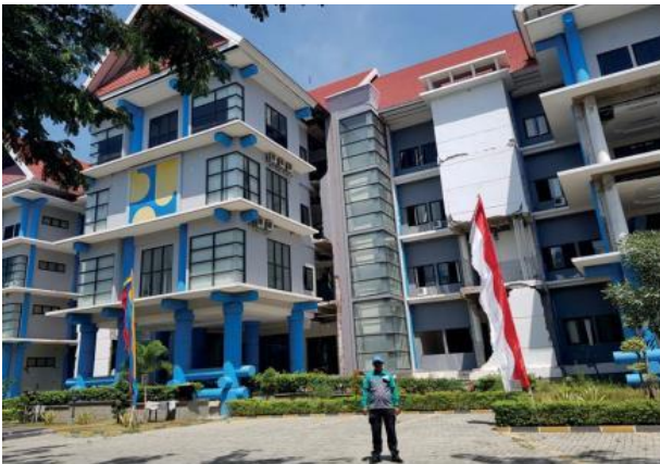
Fig. 2 – Damage in the Front of the Building
